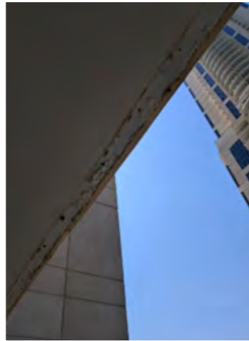
Water Leakage from Ceiling
